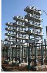
75MVAR substation capacitor bank at 150kV
